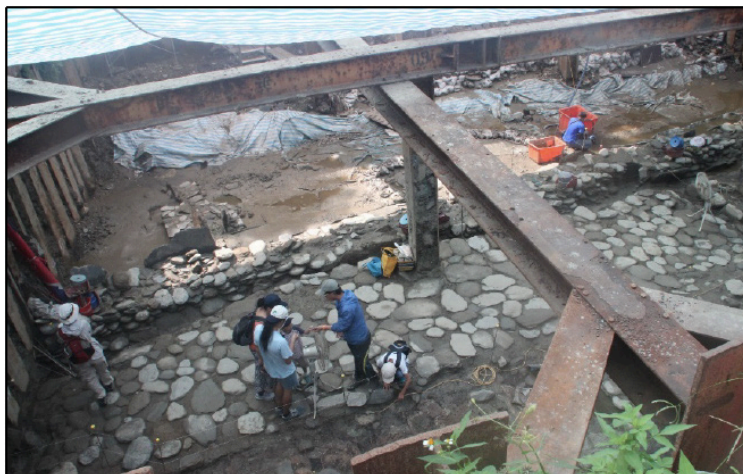
Fig. 3 Excavation at Hanben site – Public presentations - Source: the author (Picture taken on June 12th, 2016)
