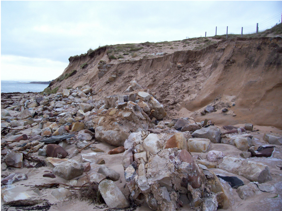
Figure 2: The salt pans one year later; undercut during a storm which caused the building to collapse onto the beach.
